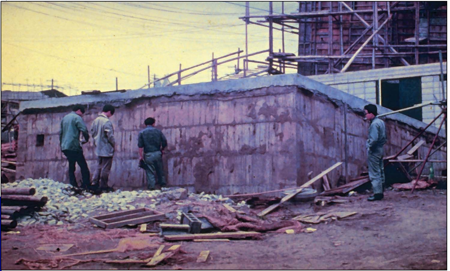
Figure 30: Floating Tank. During a 1964 earthquake in Niigata (NEE-gat-ah), Japan, the ground turned to a dense liquidlike substance, causing this empty concrete tank to float up from just below ground level. This was the first time geologists identified the phenomenon of liquefaction , which had undoubtedly occurred in other large earthquakes. Liquefaction has even lifted empty tanks up through asphalt pavement 1 and raised pipelines and logs out of the ground. 2 In other words, buried objects less dense than surrounding soil rise buoyantly when that soil liquefies. What causes liquefaction? What would happen to buried animals and plants in temporarily liquefied sediments?
